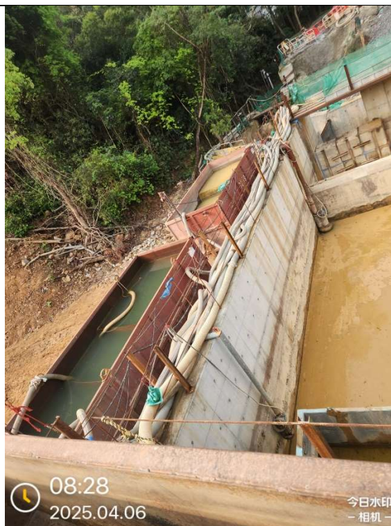
Photo 3-9 Sedimentation Basin & Tanks at Portion E3
