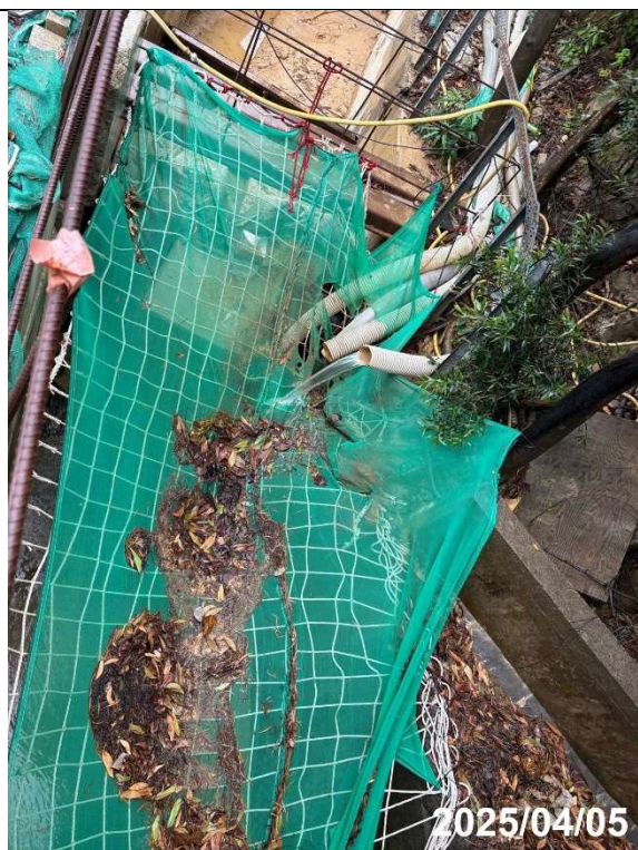
Photo 3-6 Discharge point of Silt Removal Facilities at Portion E3
